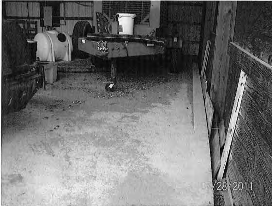
Photo 5. Photo of the portable generator staging area. Concrete pad is sloped to contain a spill.
