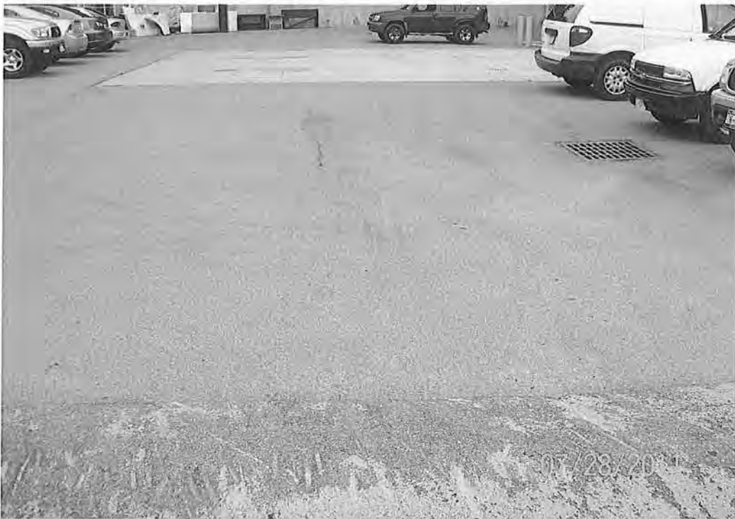
Photo 4. View of the unloading area associated with three USTs (PBS Tank #s 016, 017 and 018). Catch basin visible in picture directs flow to an oil water separator.
