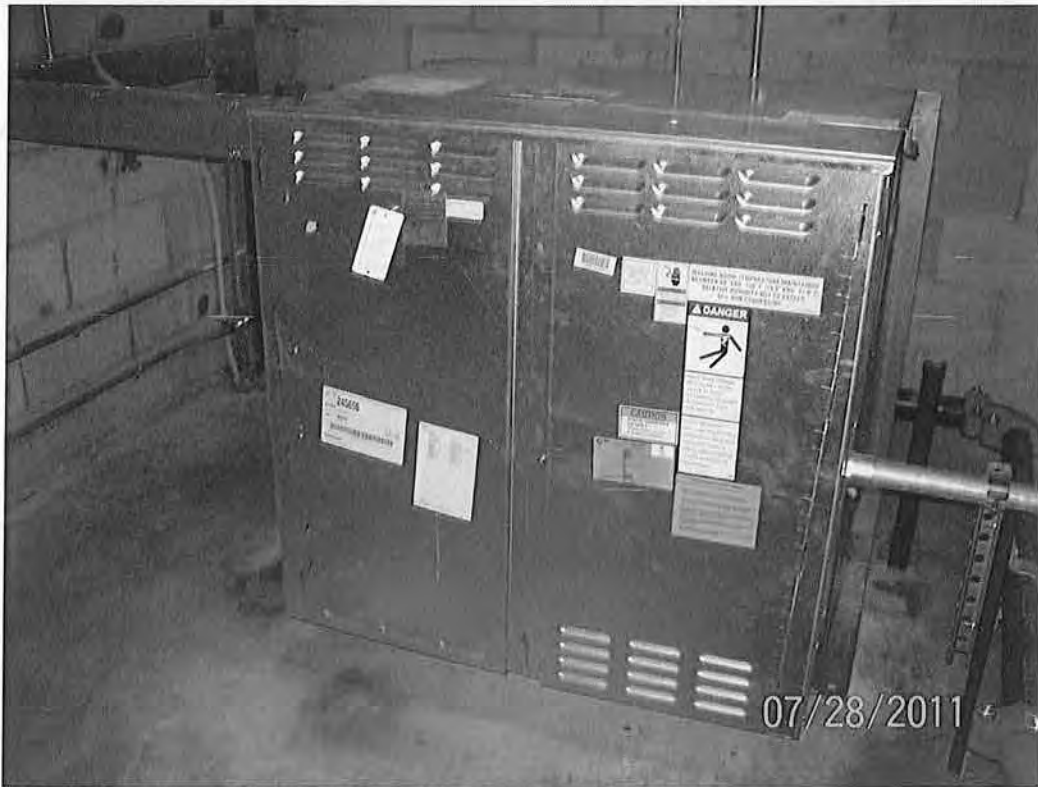
Photo 7: Photo of one of the elevator reservoirs maintained at the facility.
