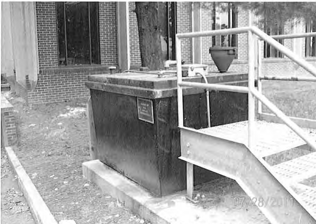
Photo 6: Photo of one of the four waste kitchen grease containers. Each of the four containers are of similar design. Two are 300 gallons in capacity and two are 500 gallons in capacity.
