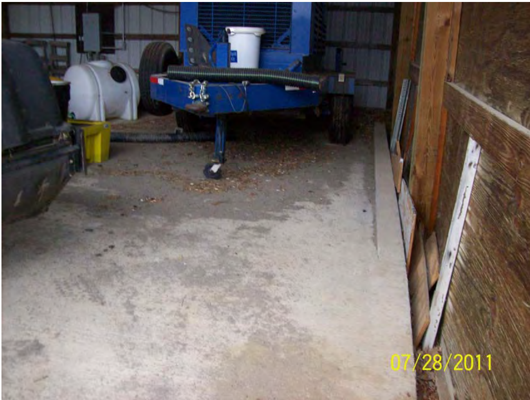
Photo 7: Photo of the portable generator staging area. Concrete pad is sloped to contain a spill.
